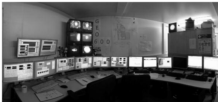
Fig.2: The main control room of GEO600.
